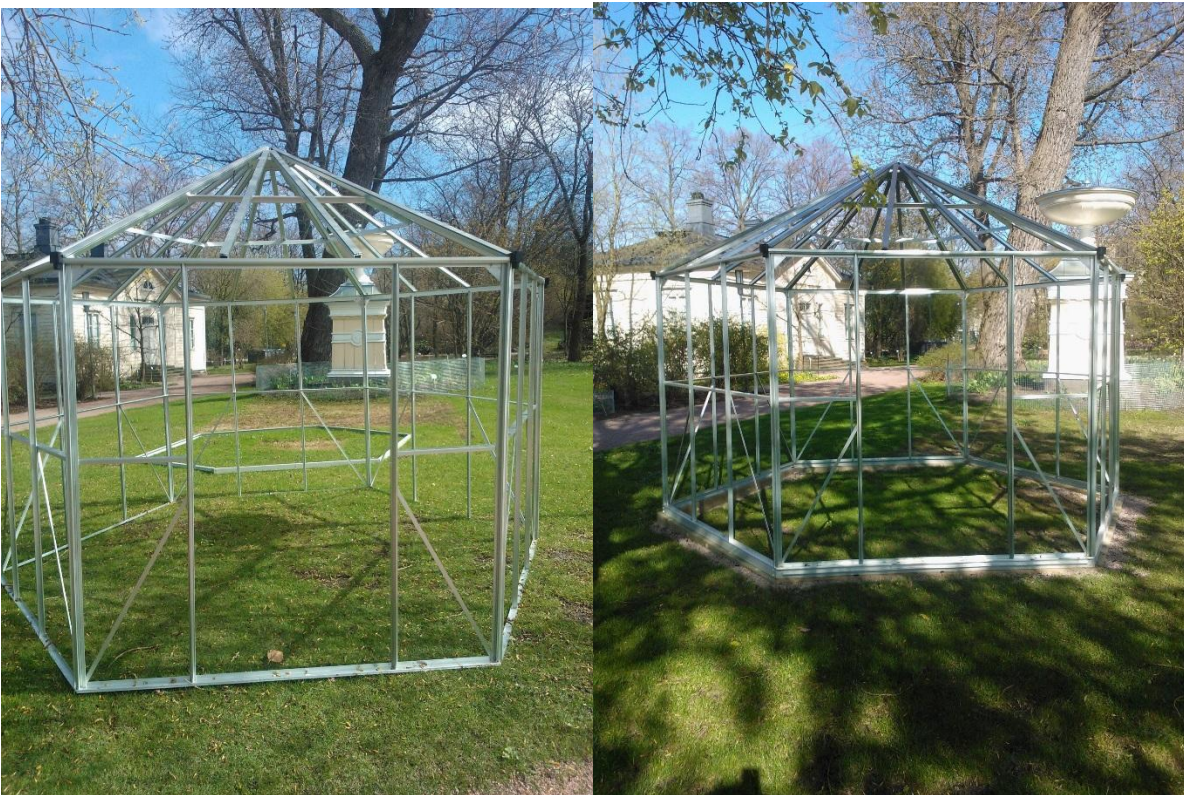
Photo 4. Different phases of ESCAPE greenhouse construction in Kaisaniemi Botanical garden, May 2015. On the left: Aluminum skeleton of the greenhouse. On the right: Skeleton elected on the plinth upon. Photos: Sanna Laaka-Lindberg
