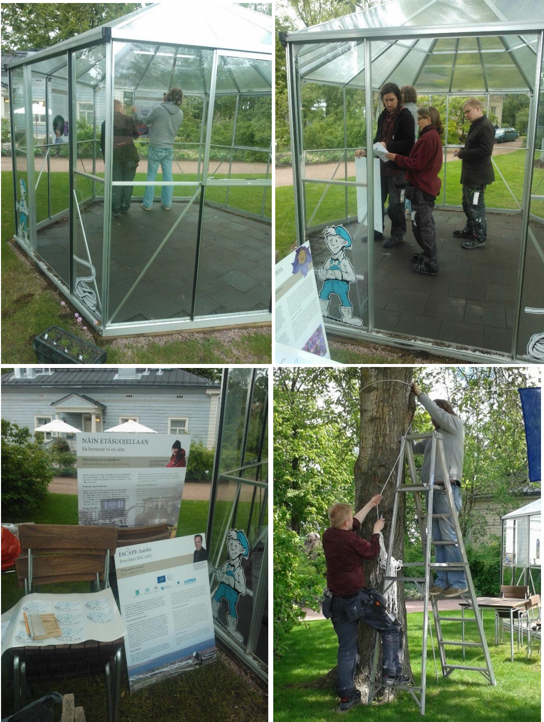
Figure 5. Erecting ESCAPE ex-situ exhibition in Kaisaniemi Botanical garden in early June 2015. Up on the left: glass walls of the greenhouse and concrete slab floor finished. Up on the right: Placing the posters. Note the cartoon gardener character on the outer wall by the door. On the left below: The parts of the exhibition display waiting to be placed. On the right below: Tweaking the LIFE flag outside the exhibition greenhouse. Photos: Sanna Laaka-Lindberg 2015, except on the right below: Kirsi Hutri.
