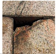
Broken corner of a granite block from the wall of the Helsinki Cathedral.
